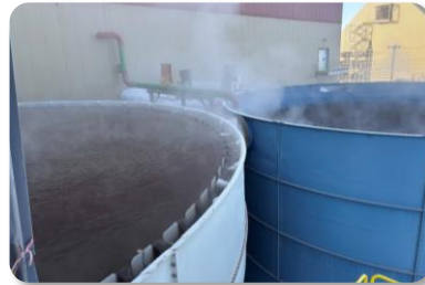
Thickener and process water tanks
