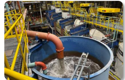
Recirculated (teeter) water tank
