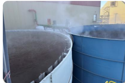
Thickener and process water tanks
