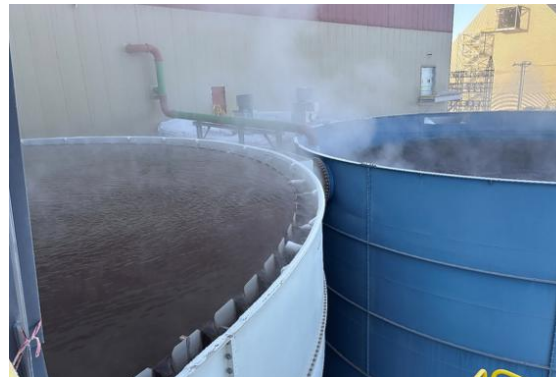
Thickener and process water tanks
